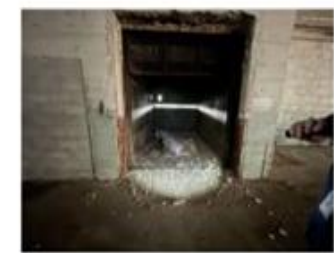
B - Deteriorated Lintel Elevator 9
