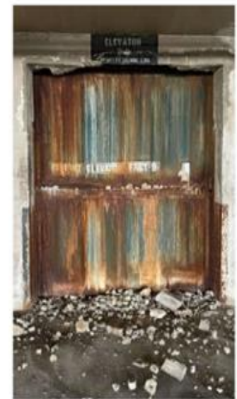
C - Deteriorated Lintel Elevator 9
