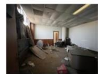
F - Buildout at north of floor and rubbish
