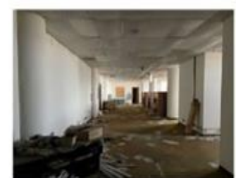
E - Buildout at north of floor and rubbish
